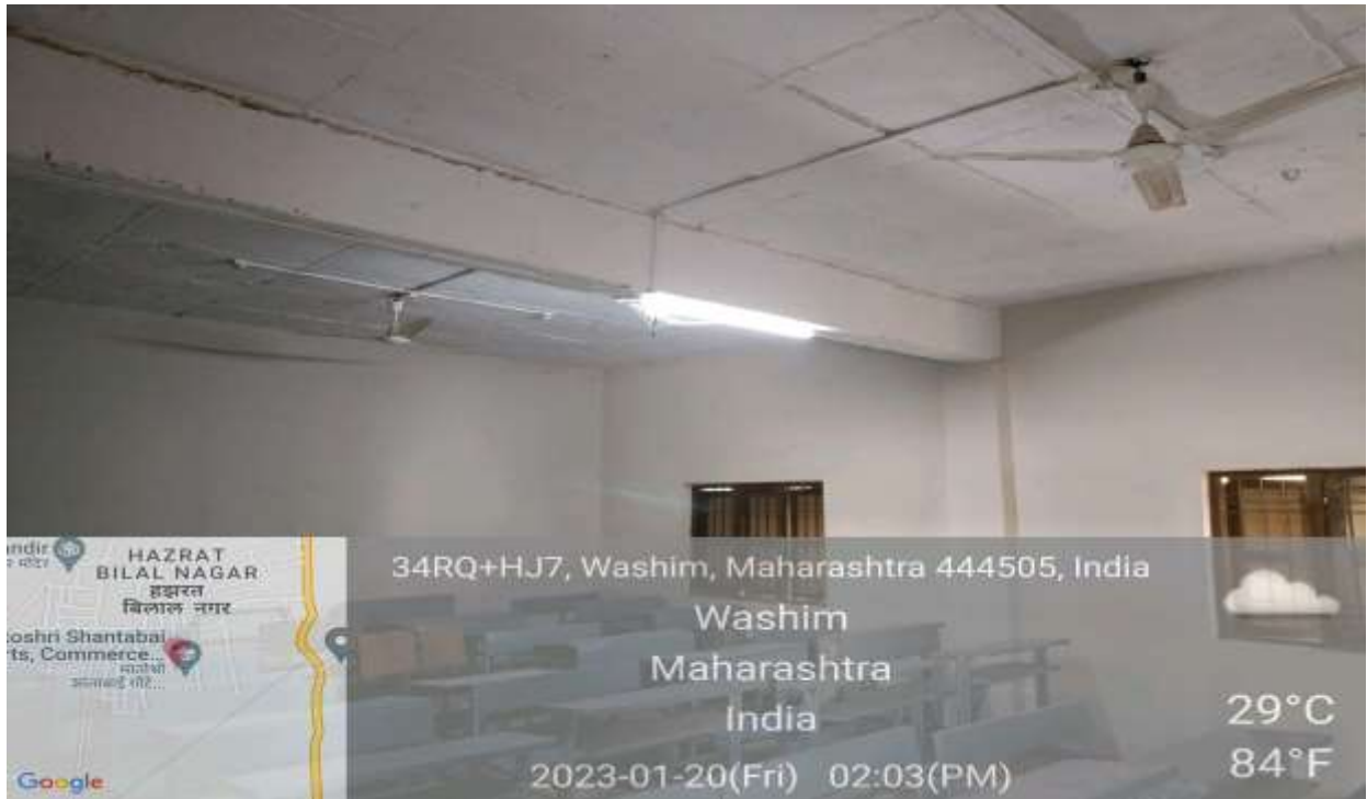
Light & fan In all Class Rooms
